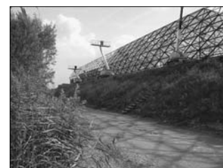
Fig 5C: Acoustic Barrier, ONL [Oosterhuis_Lénárd] 2004, Building site progress, 15 September 2004, the Cockpit will connect to the left end
